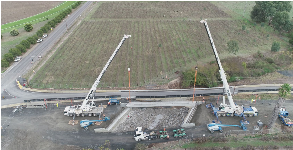
Erecting girders at Clare site, Max Cranes from Pt Pirie & Pt Augusta) Concrete from Clare Concrete, Hallett Pt Pirie. Demolition, haulage of waste undertaken by SC Heinrich (ex Clare)
