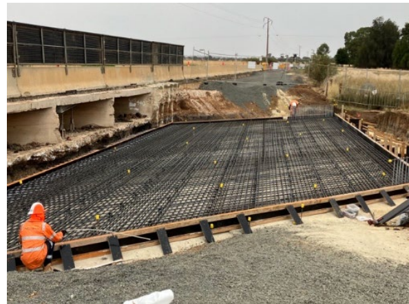
Ngurra civil adding the final touches to a base slab before concrete arrives (Eudunda).
