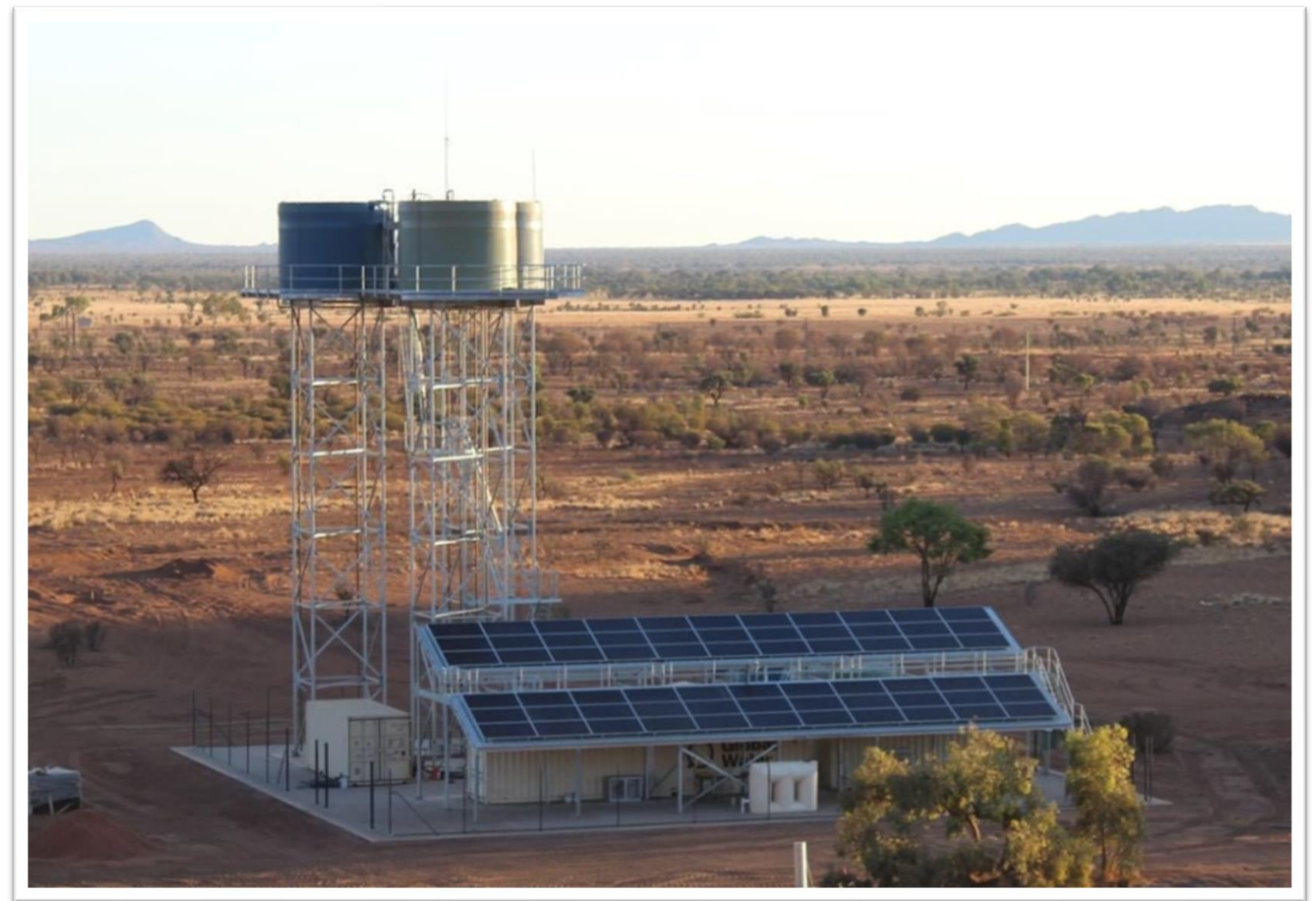
Fusco Constructions completed works for the SA Water Nyapari, Kanpi and Murputja Water Upgrade
